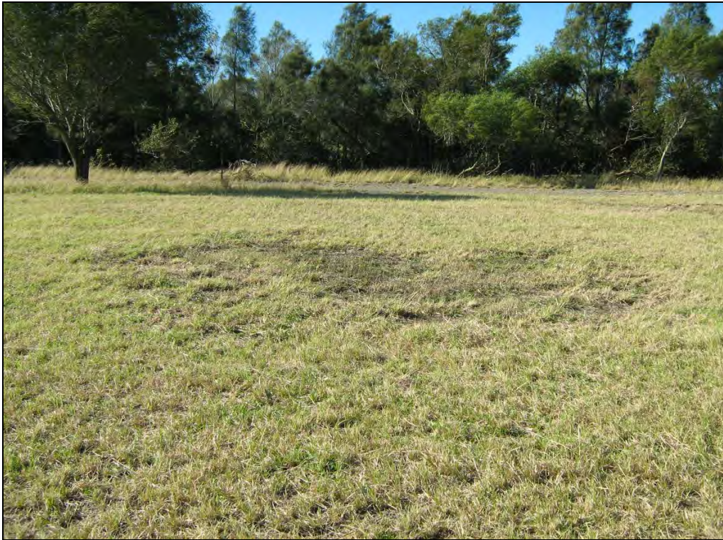
Figure 2: Localised surface depression in southern portion of the site (looking east June 2008)
