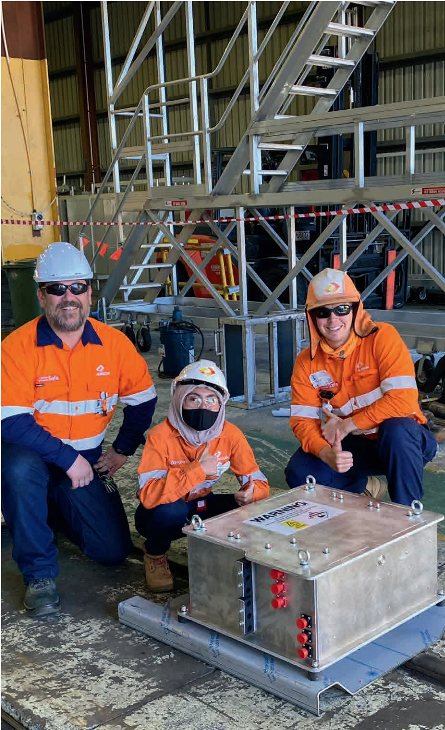
The project team taking delivery of a Li-ion battery before installation, allowing reactivation of AESS technology on one of our diesel electric locomotives.
